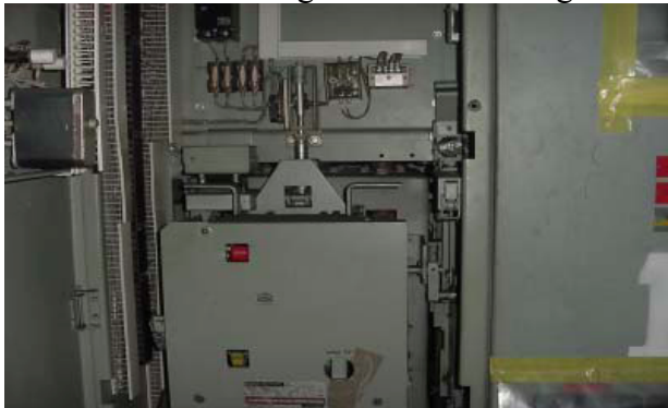
Normal breaker arrangement at a switchgear
